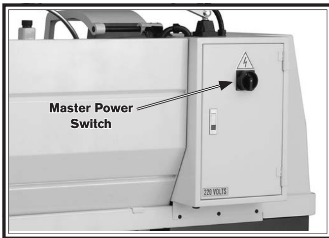
Figure 28. Location of the master power switch.
